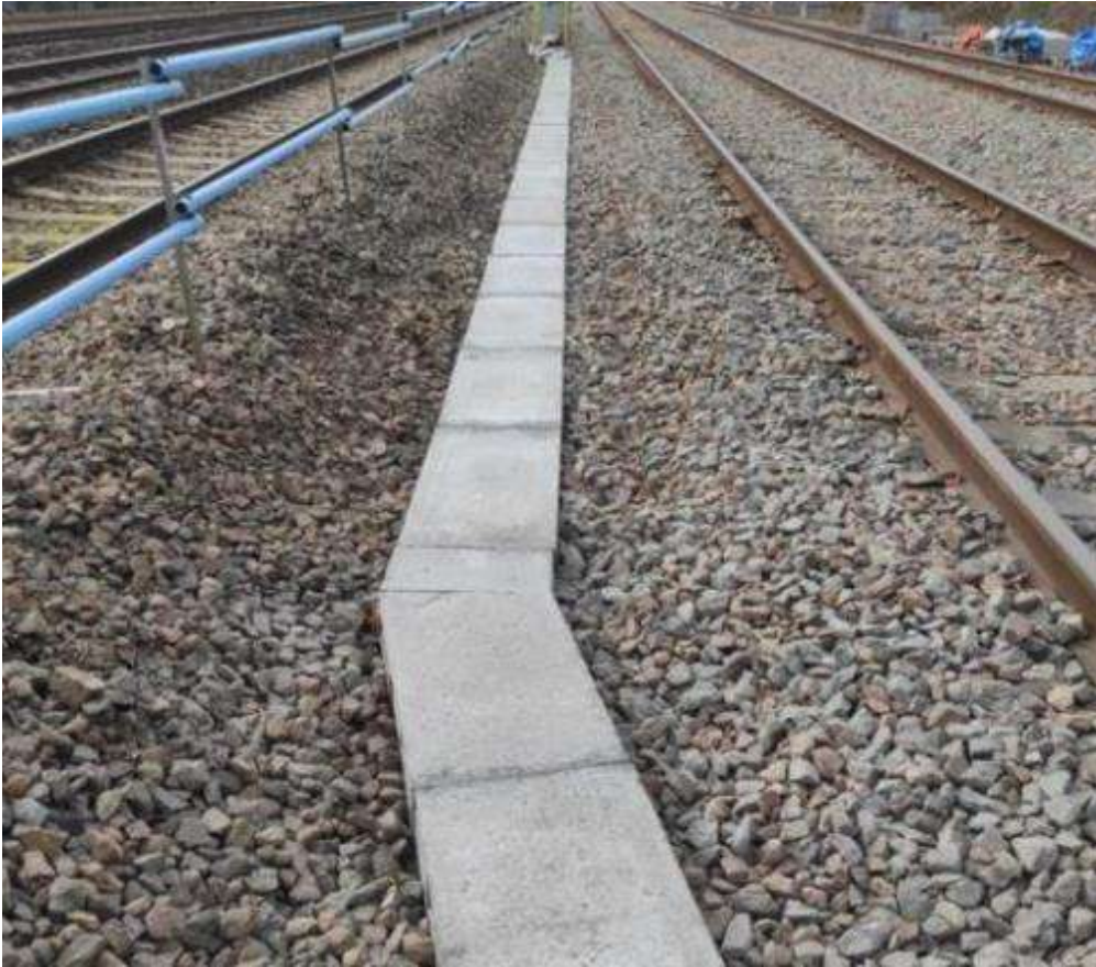
Figure 5-12 Example of Concrete Cable Troughing
